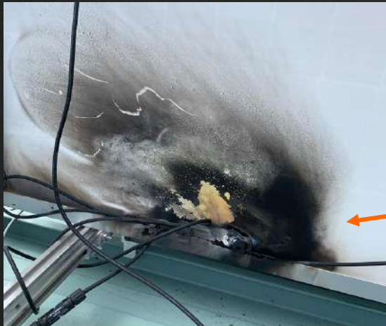
Visual Impact: Silicone smoking out, discolored backsheet, melted enclosure
