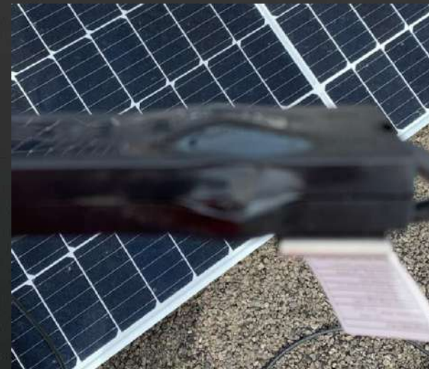
Visual Inspection: Enclosure bubbling
